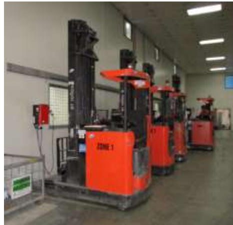
Figure 12: Reach Trucks parked in Battery charging area at end of shift
